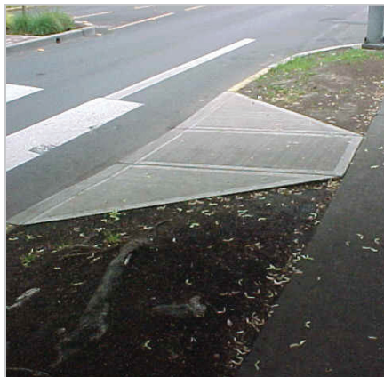
Sidewalks compliant with ADA requirements guarantee that all citizens can move throughout the Study Area
