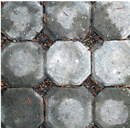
Porous pavement helps stormwater to more easily filter into the ground surface
