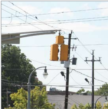
Overhead utility wires in the study area clutter the view in many places
