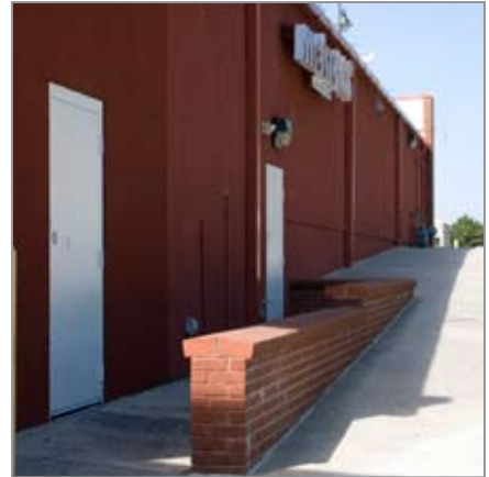
Buildings should never present a blank wall to the sidewalk
