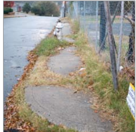
Neighborhood sidewalk repairs are critical for safety, mobility, and perceptions
