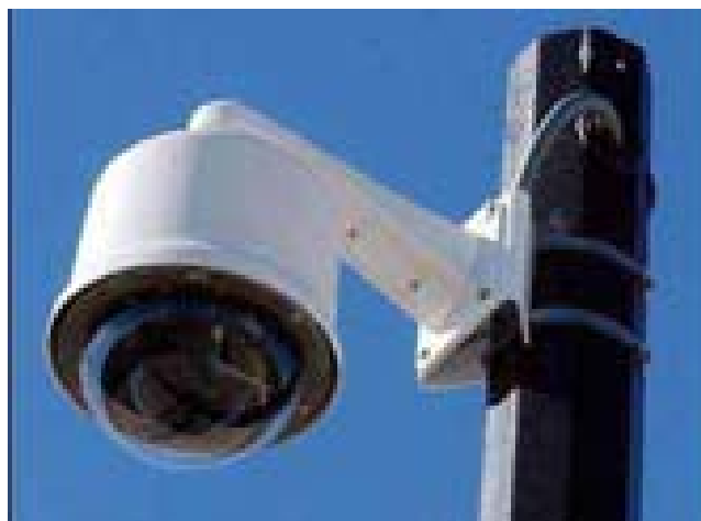
Security cameras should be installed along Boulevard
