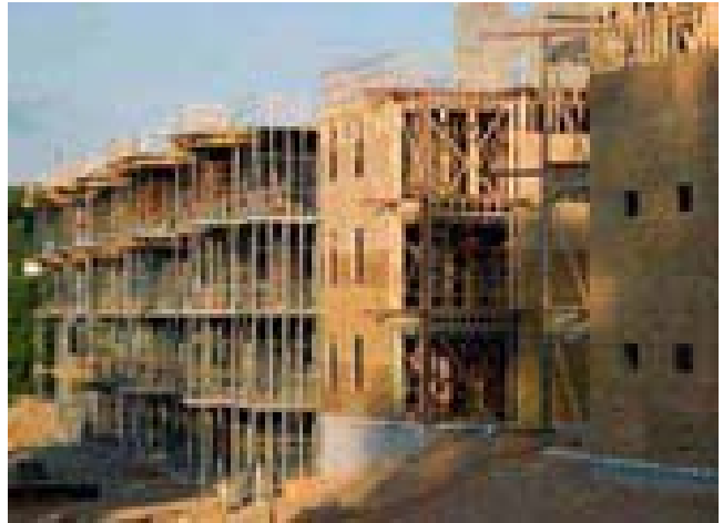
New residential development under construction between Glen Iris Drive and the proposed Historic Fourth Ward Park
