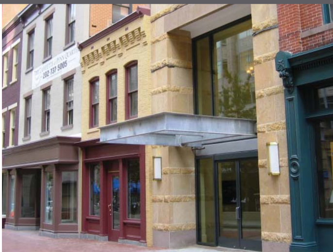
CANOPY STRUCTURE AND MATERIALS Cantilevered from a heavy stone base, this canopy provides a simple and strong solution to inclement weather for this entry.
