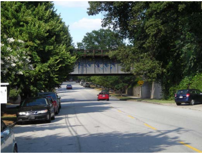
The existing BeltLine alignment passes over Ralph McGill in a bridge which accommodates only a double rack of transit. An additional pedestrian bridge will be necessary
