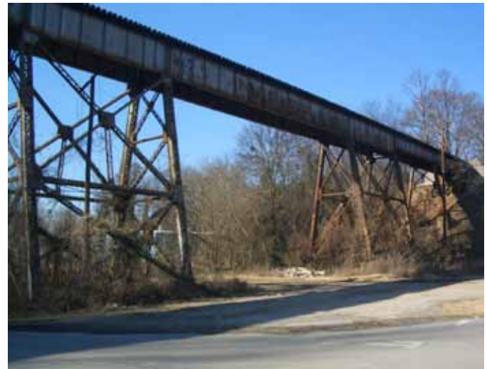
Transportation infrastructure, like this CSX railroad trestle, has a significant influence on the character of Subarea 10.
